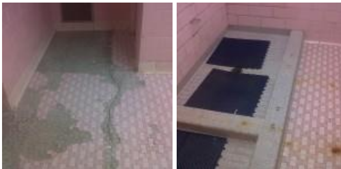
Before: Deteriorated, unsightly 2 nd floor shower room tile harbors mold & germs – and leaks water to lower levels.
