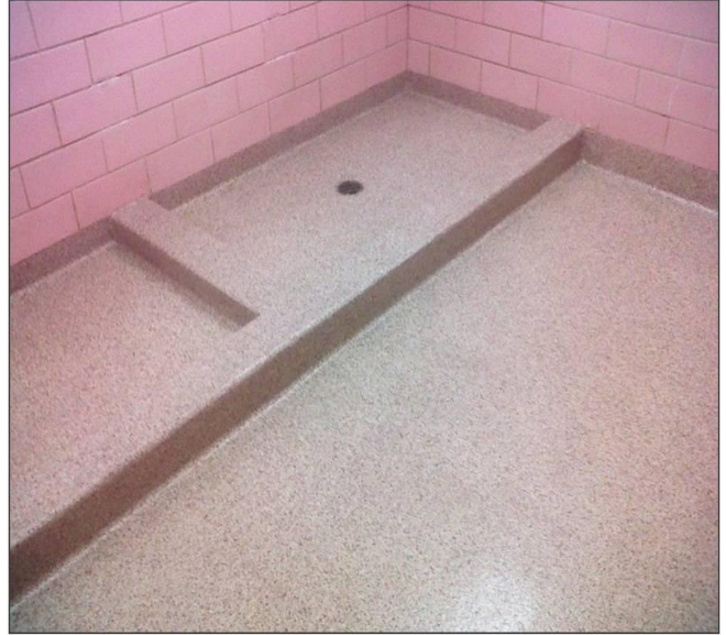
After: Gorgeous, functional and safe FloroCryl Chip flooring, skillfully installed by Industrial Coatings, Inc.
